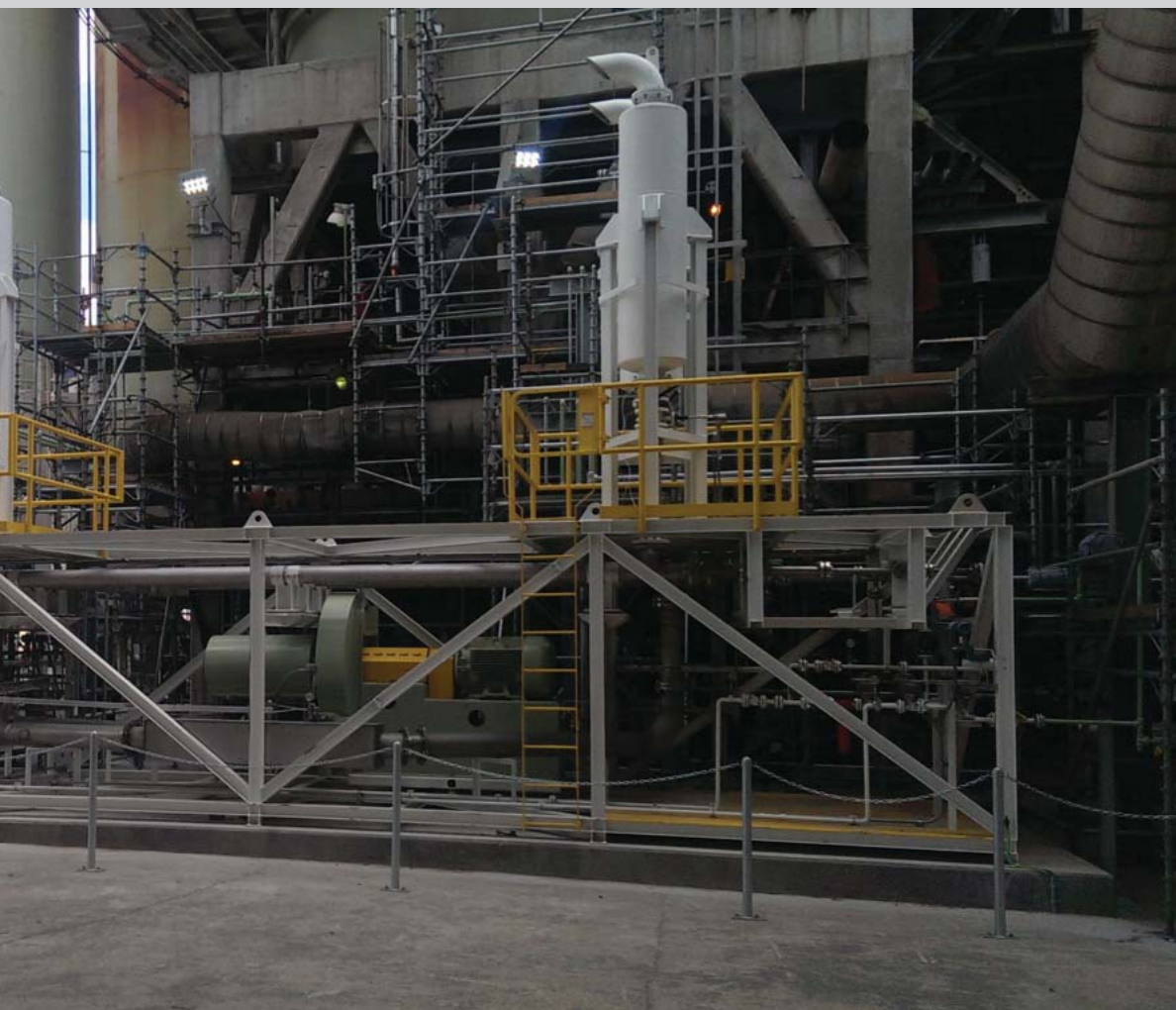
Image1. Continuous Catalyst Withdrawal (Mark-I) Installation – Marathon Petroleum Refinery, Garyville, LA
