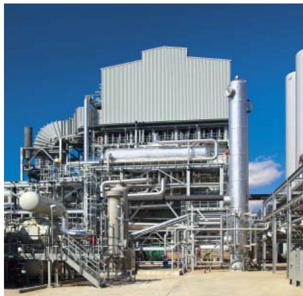
– Air Products' industrial gas facility at Convent, Louisiana, USA.
