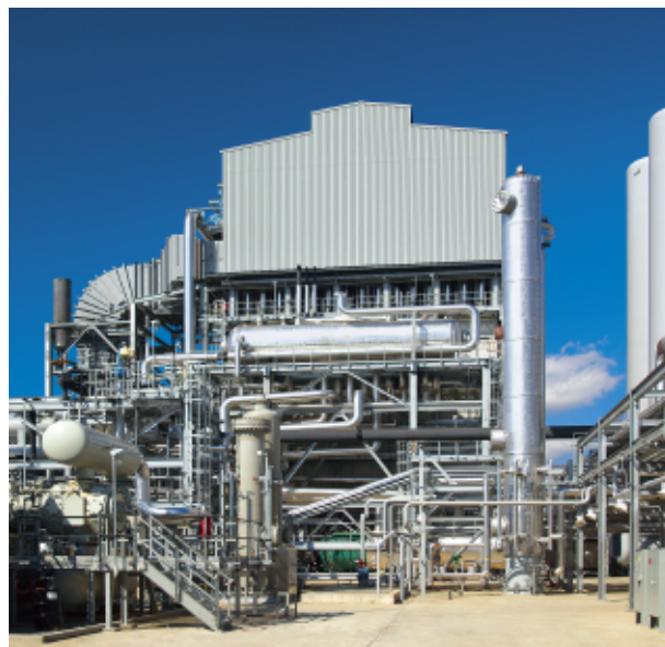
– Air Products' industrial gas facility at Convent, Louisiana, USA.
